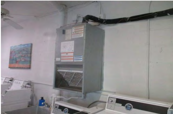
21 Laundry Room HVAC
