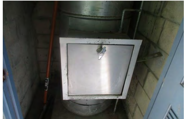
22 Trash Chute Overview
