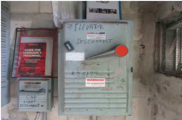
29 Elevator Shut Off
