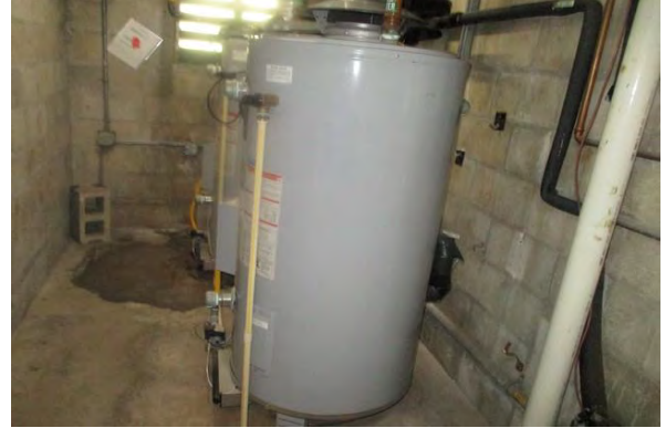
12 Water Heater Overview
