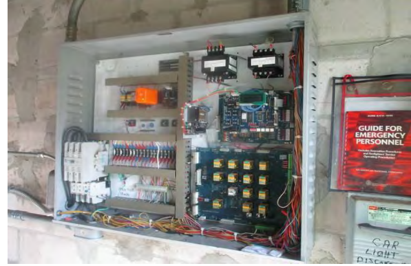
28 Elevator Control Board
