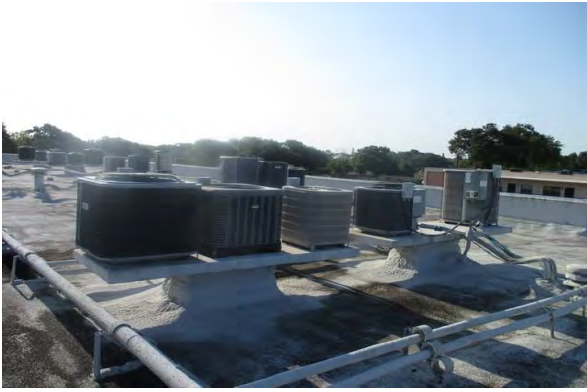
9 HVAC Stand/s Overview
