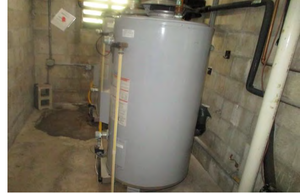
12 Water Heater Overview
