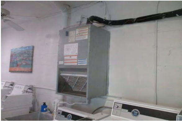
21 Laundry Room HVAC
