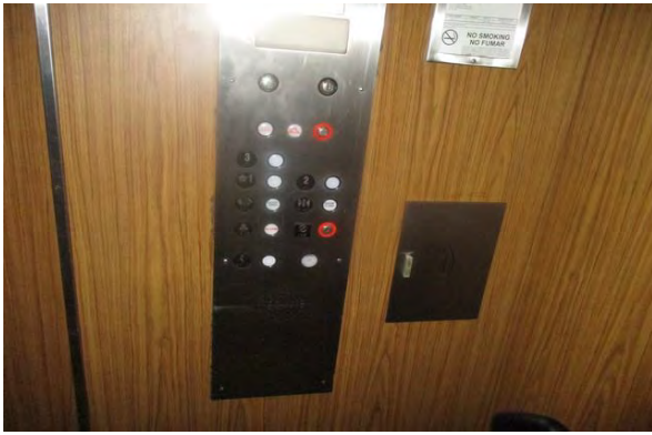
33 Elevator Control Board
