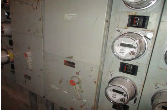
27 Main Shut Off Overview
