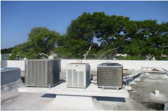
5 HVAC Stand/s Overview
