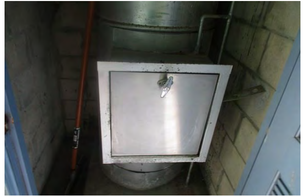
22 Trash Chute Overview
